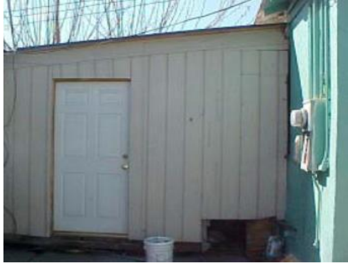
Construction without building permits
