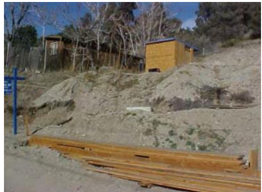
Grading without permits
